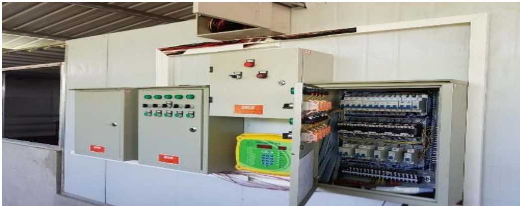
Gambar 4. Control panel exhaust fan (blower) full otomatis
